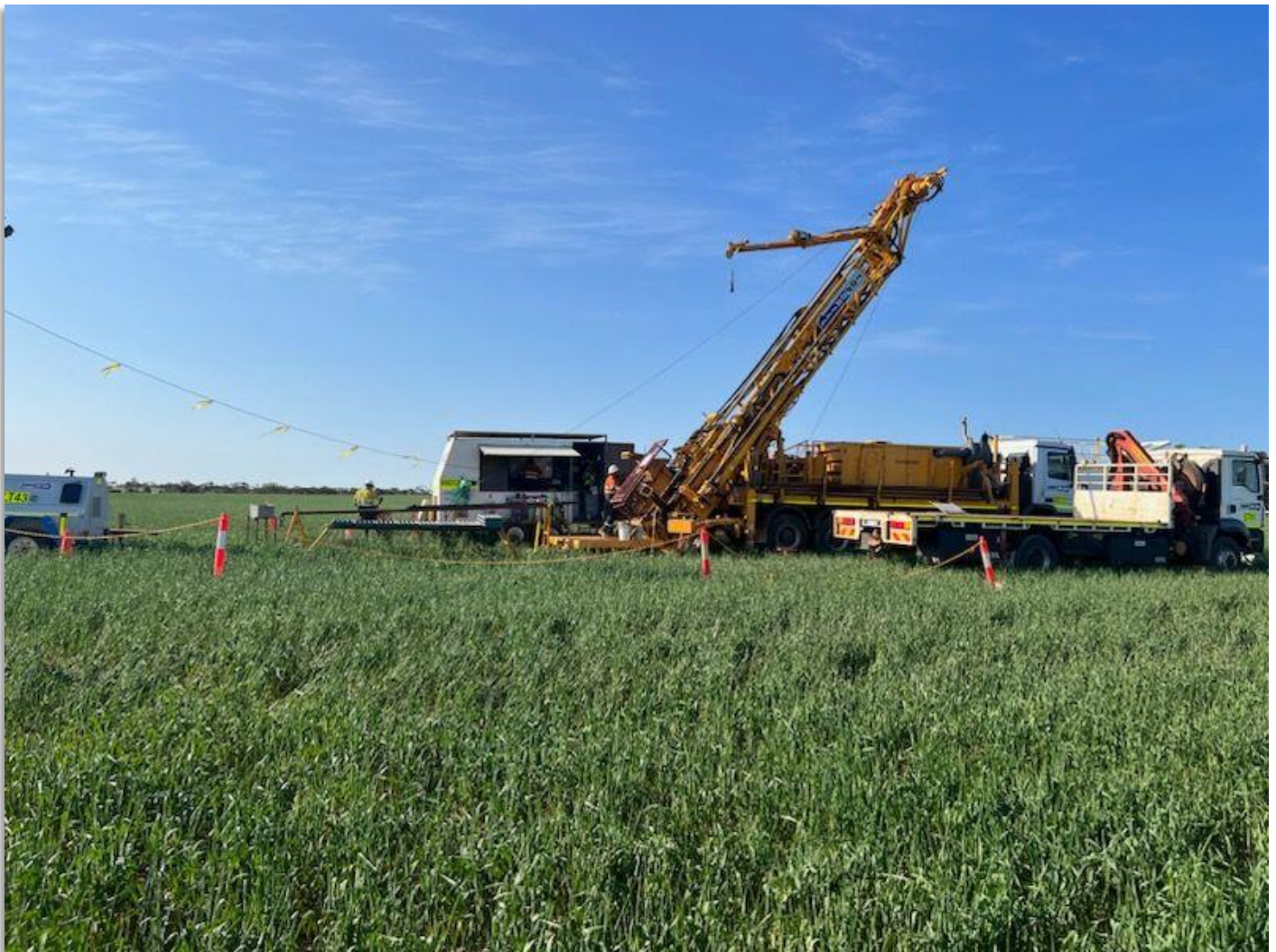
Figure 1. Topdrill diamond rig set-up to drill at the Salmon Gums Gold Project.
